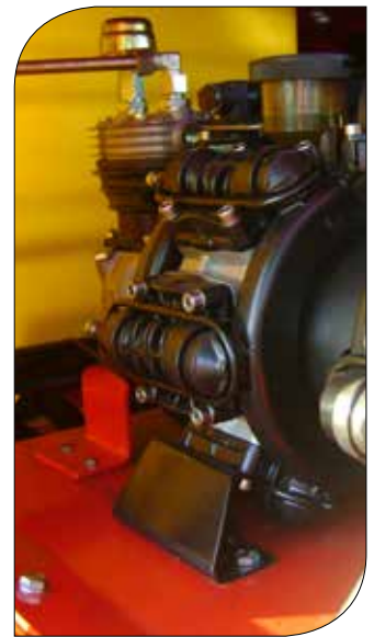
Compressor behind pump
