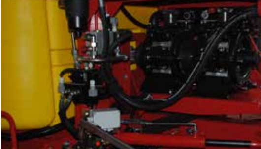
Accessible pumps so that maintenance can be performed easily.
